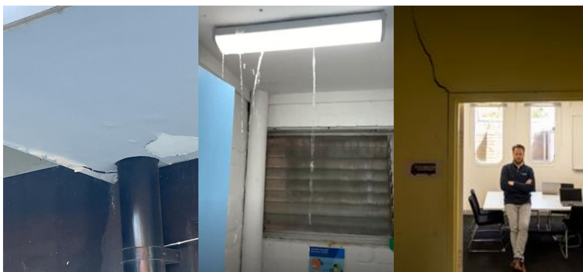
Disrepair of the roof at IPC Health in Hoppers Crossing causes the building to flood during heavy rain. Rainfall leaks through lights have led to emergency closures at CoHealth in Collingwood. Source: Infrastructure Victoria, Investing in community health infrastructure .
